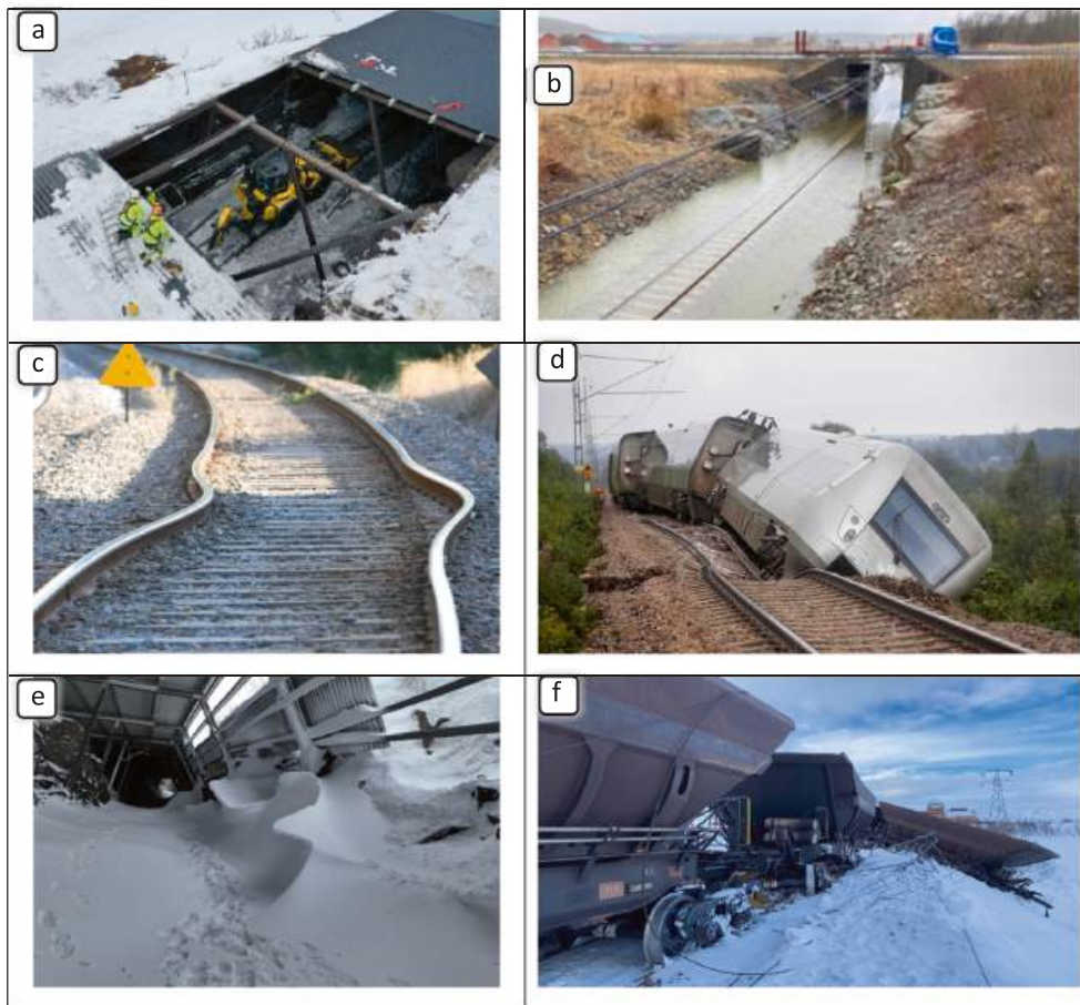
Fig. 1. Examples of climate-related stressors and resulting failures in railway infrastructure. Panels illustrate how climate hazards (stressors) such as snow accumulation (a, e), flooding (b,d), extreme temperature (c,f), and extreme snow and wind (a, e) can lead to infrastructure failures including overload, erosion, rail buckling, and derailments. These examples highlight the vulnerability of railway systems to evolving climatic extremes. Photos
